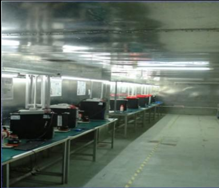
RF SHIELDING ROOM
